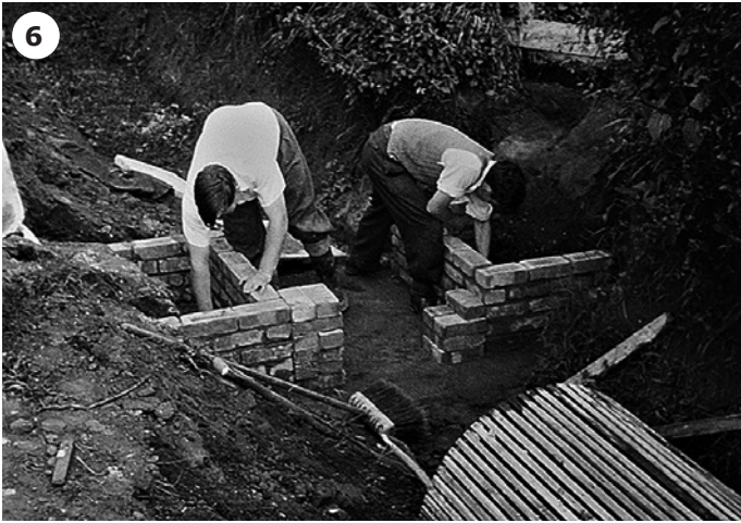
Pic 6: Building an ornamental bridge in the First School garden c1957 with Len Jarvis on the left, learning what was to become his trade for the rest of his working life.
