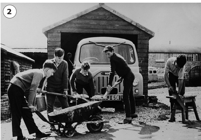
Pic 2: First School pupils building a minibus garage. Peter Moss, Paul Prentice, Rodney Nudds, John Housden and Fred Hill. The pupils made the shed for the school's mini bus on the top field, with Mr Freeman the woodwork teacher taking charge. It showed what skills the pupils had learnt in class and gave something extra for the school to benefit from for years to come.
