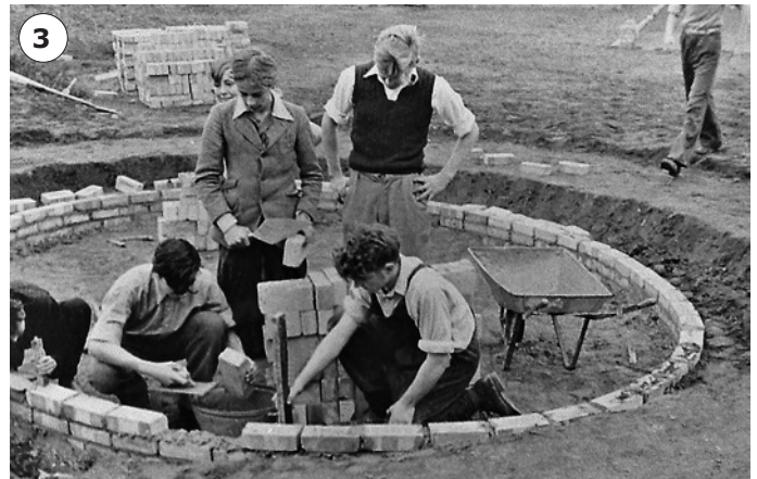
Pic 3: These pupils built a paddling pool, sand pit and thatched shelter to sit in when the sun was too hot. Here we see sixth formers Len Jarvis and Jim Staughton laying concrete for the bottom of the paddling pool while being watched closely by younger pupils in 1952-53. Len was to become a Master Builder with his own business specialising in renovating old properties.
