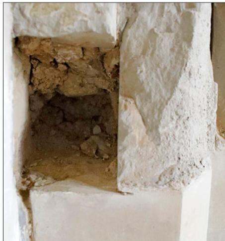
The far from solid Bath stone columns making up the chancel arch – the layers of flaking clunch are to be replaced.
