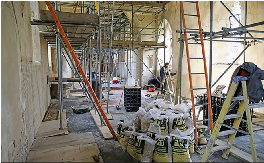
State of play in St Denis' at the end of January – much scaffolding and much work to be done to remove the old plaster (now in the plastic bags) and re-plaster the walls with a traditional lime putty mortar.
